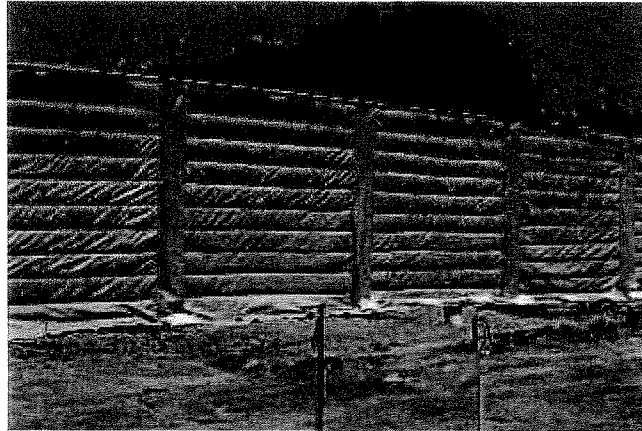
FIGURE 7. Noise Blanket as Barrier Wall
