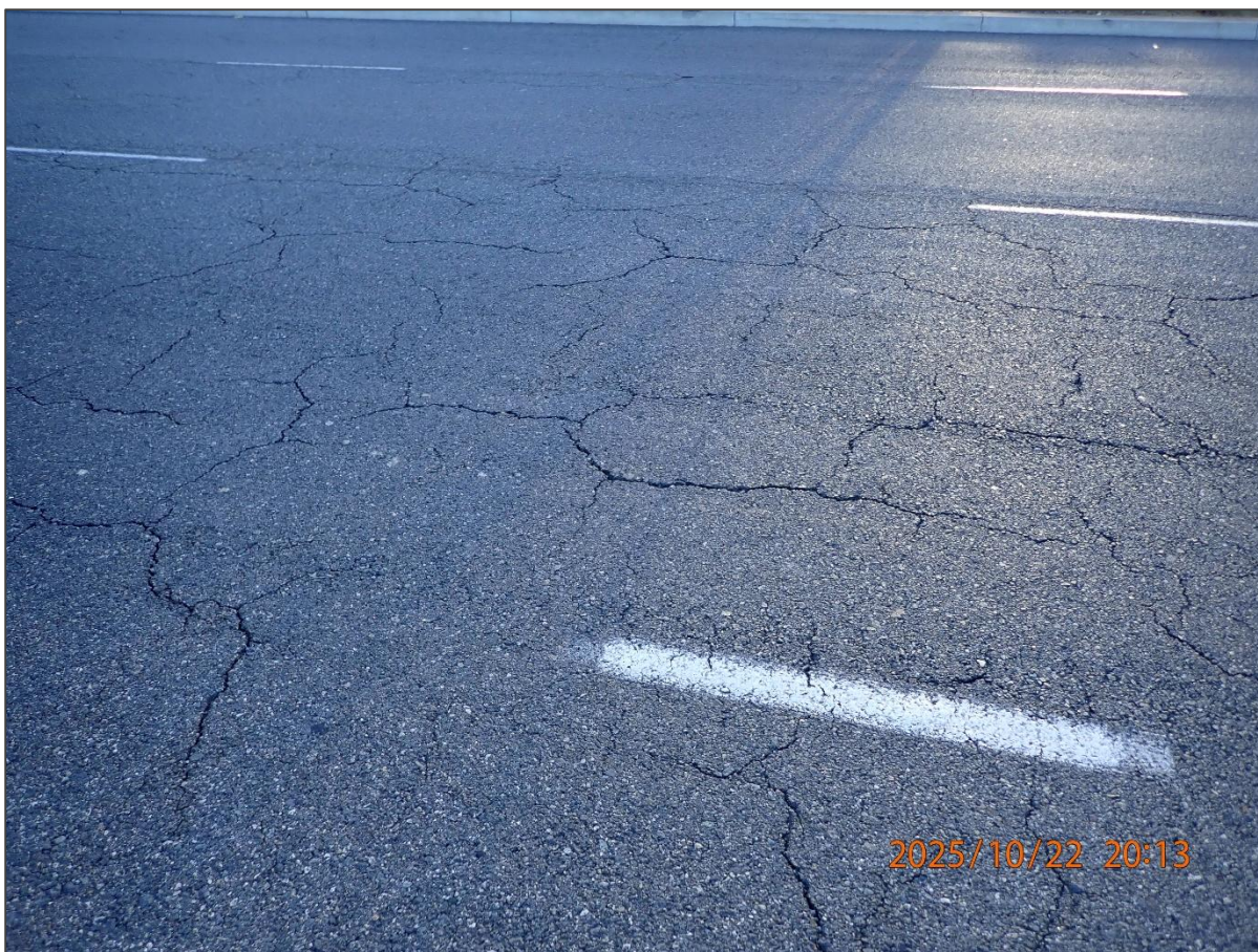
Figure 8 – 2025 Wide, Fully Interconnected Cracks
