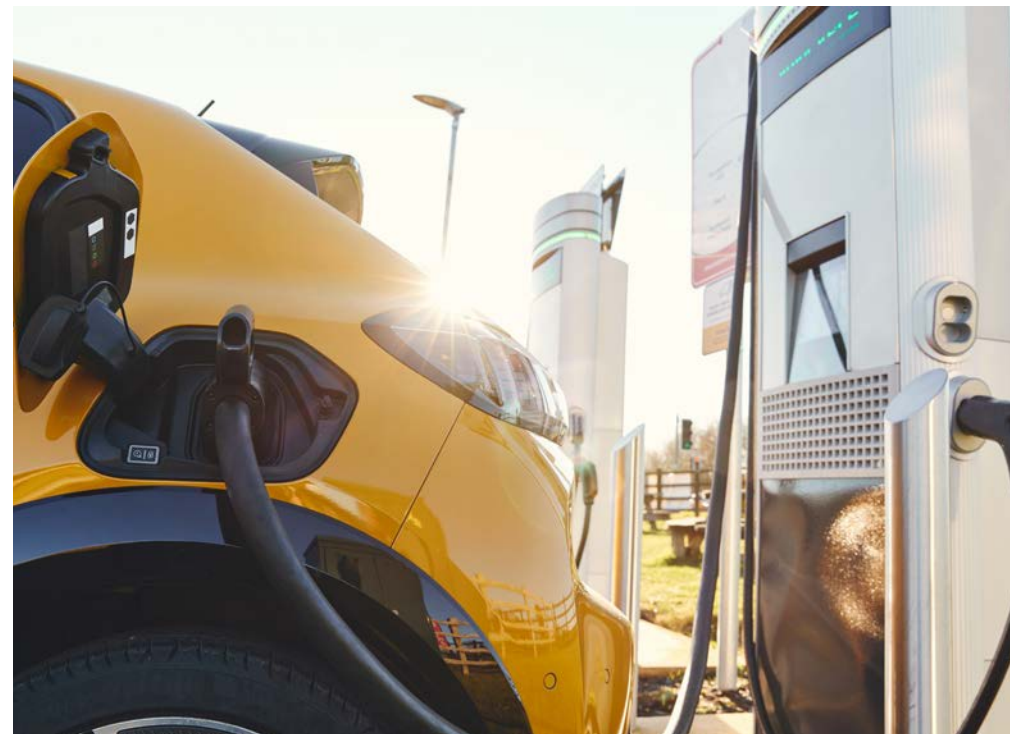
EV CHARGING STATIONS
