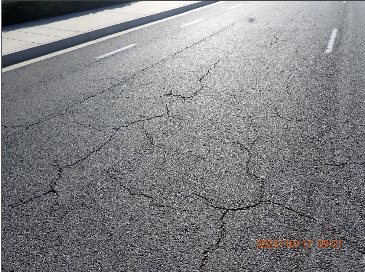
Figure 7 – 2023 Tight/Narrow, Partially Interconnected Cracks
